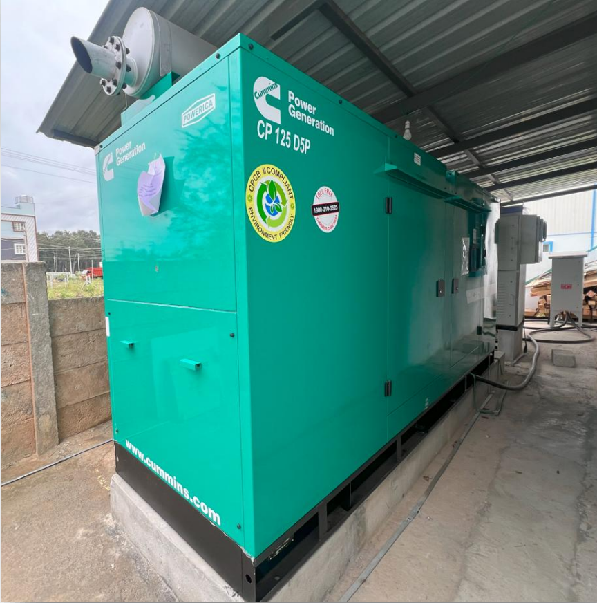
Diesel Genset Capacity – 125 Kva
