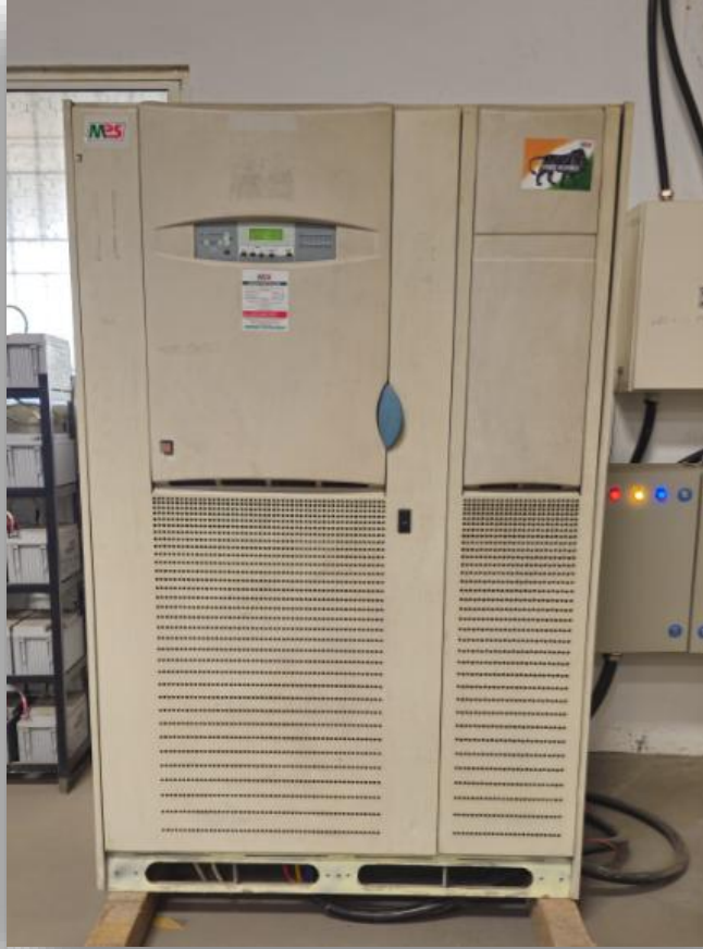
UPS Back up Capacity – 100 Kva
